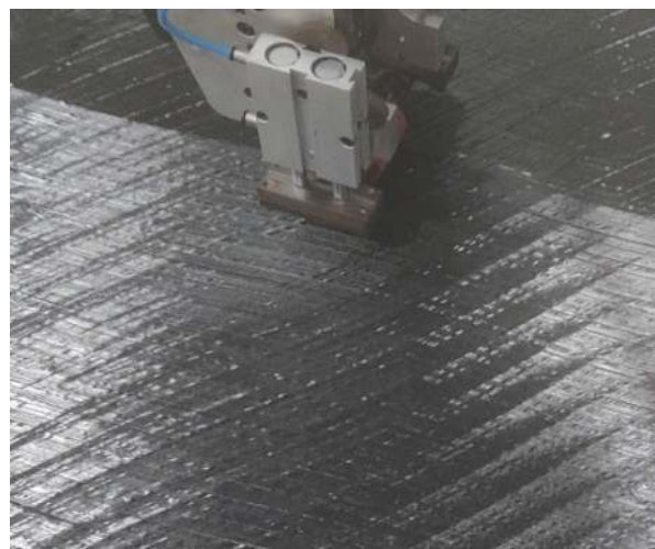
图5 8丝数EM118碳纤维增强树脂预浸料窄丝(3.175 mm)自动铺放 Fig. 5 Automated fiber placement of 8-thread EM118 carbon fiber reinforced resin prepreg narrow tow (3.175 mm)
